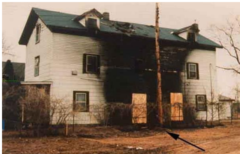
Fig. 1.2 Fire scene showing a 'V' shape pattern indicating the point of origin towards the foot of the 'V'
